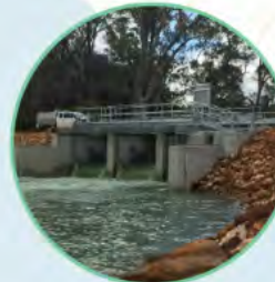
Regulators will help us to move water onto the floodplains and hold it there before opening the regulator to return water to the river. Regulators will include fishways to help native fish on their journey.
